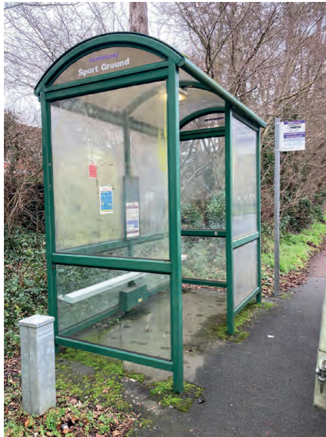
Bus shelters in residential development provide protection in inclement weather and should be durable and vandal proof
